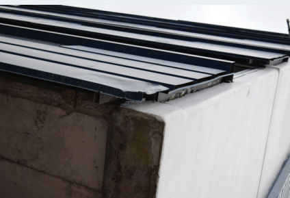
Facade sheet metal bent
